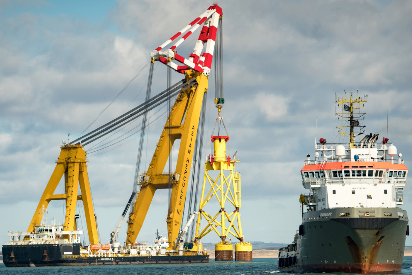
Installation of a suction bucket jacket foundation for the Aberdeen Offshore Wind Farm by the floating sheerleg crane Asian Hercules III.
